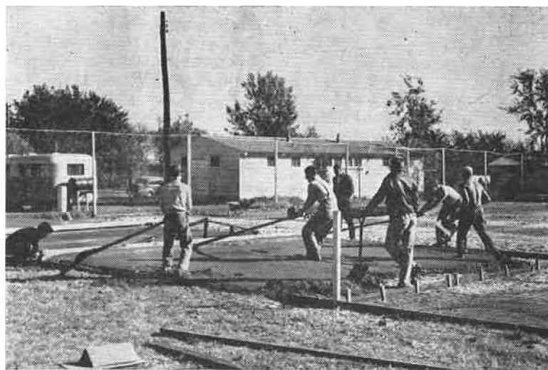
The Y. C. dream of all-weather tennis courts begins to take form as the first section of concrete is poured. Pictured are some of the boys doing volunteer work. The never-tiring Coach Tonkin is supervisor of the project.
